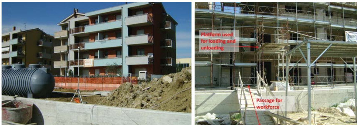
Fig. 3. View of the construction site with one of the receivers (a); close-up view of the platform with localization of the hazardous area (b).
