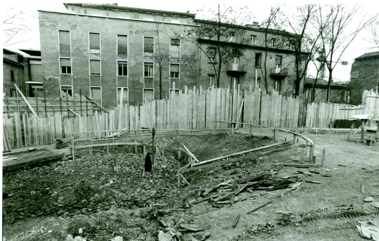
Bologna, the Giardino del Guasto as a building site during the completion of architect Filippini project.
