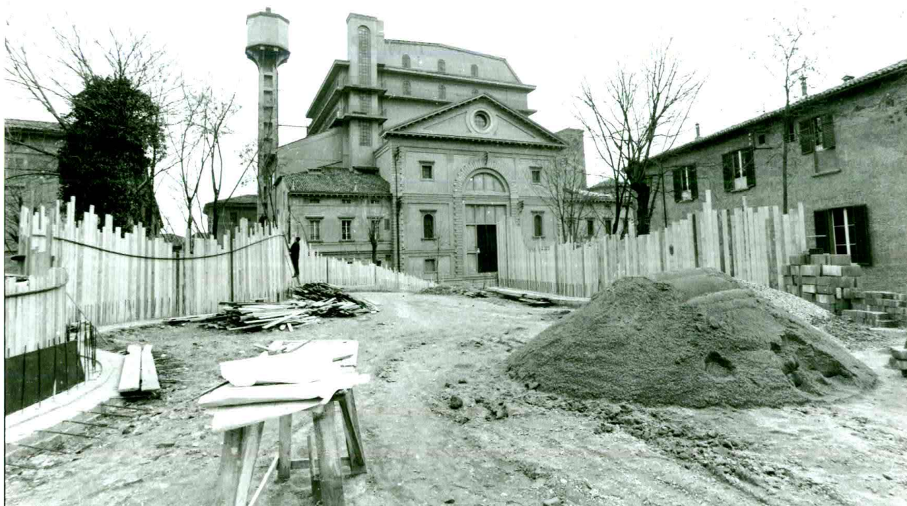
Bologna, the Giardino del Guasto as a building site during the completion of architect Filippini project.
